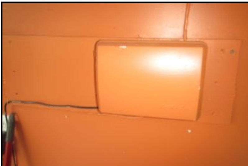
Sprinkler timer noted
