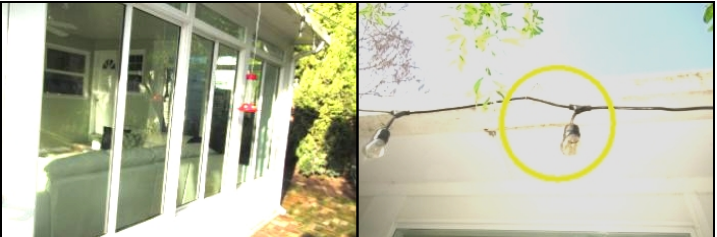
Water stains present at the overhang.
